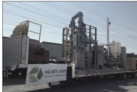
Electric Heater (pilot)
